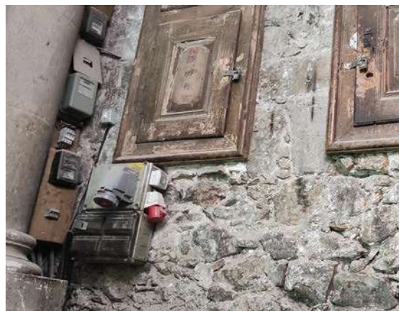
Fig. 2. Electrical switchboards and meters near the main entrance of the church.
