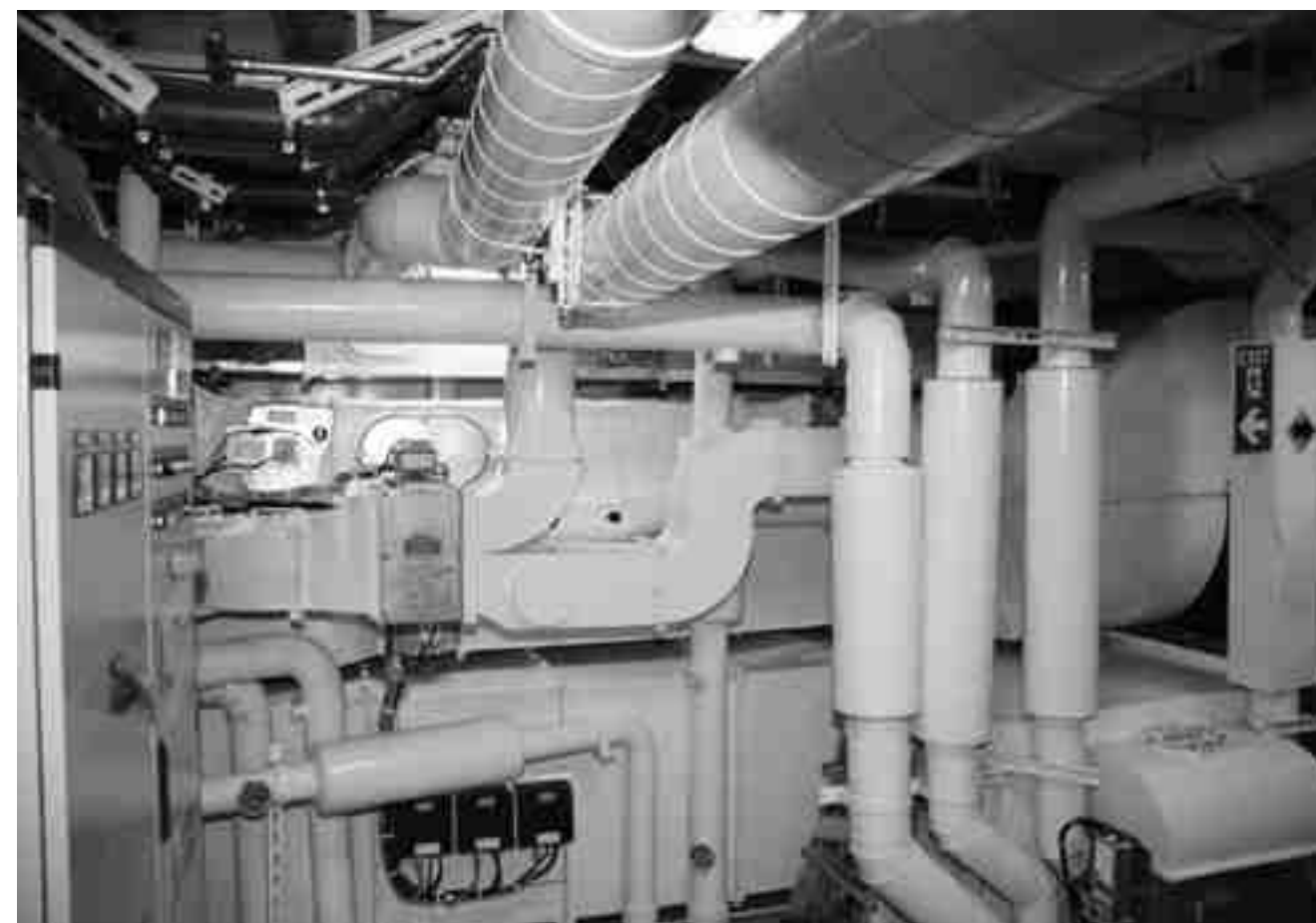
Impianto HVAC – Macchinari in AC station
